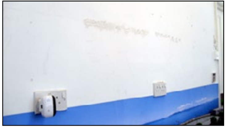
Nicely untreated wall with cover removed from live socket at the far end.
