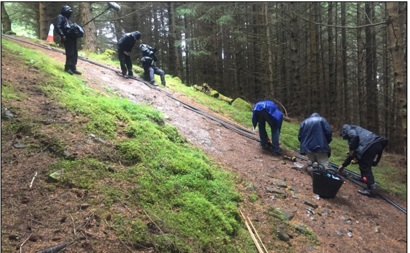
Above: Team D, Laying A Challenge Section On What Became 'Heart Break Hill' While Building A Rack & Pinion System (Photo Credit: Paul Tyer)
