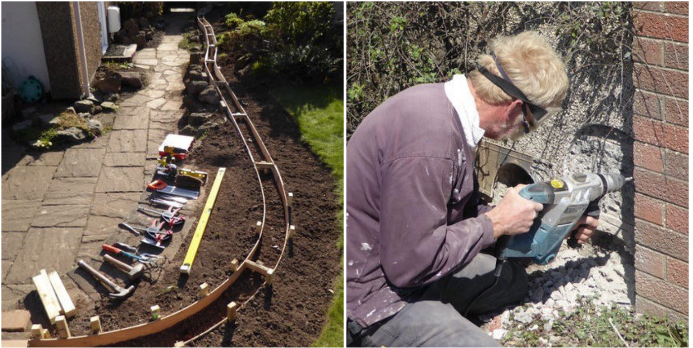
Above Left: Foundation Preparations For The New Railway Line Above Right: Drilling Out The New Tunnel Portal
