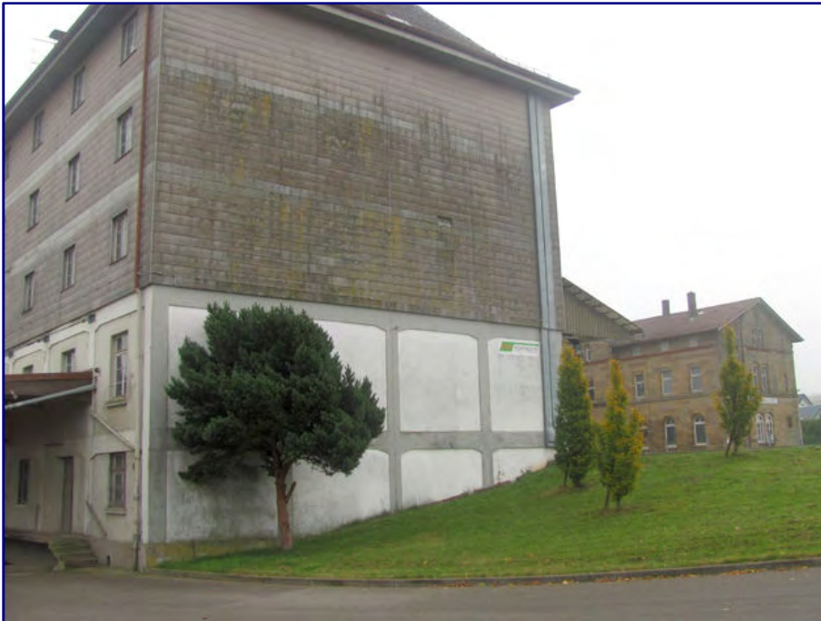
From this perspective, the hillside location can be seen well, which can also be illustrated with the kit. In the background you can see the reception building of the station Eckartshausen-Ilshofen, which is also offered as a model. Photo: Stefan Laffont
