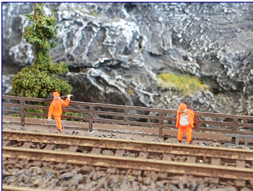
Sersa's track construction team is working hard to make the line passable again on both tracks.
