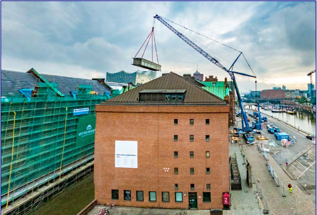
In the early morning hours of 15 July 2020, Europe's second largest mobile crane lifts the 39-tonne bridge 40 metres above the storage building. Photo: Miniatur-Wunderland.
