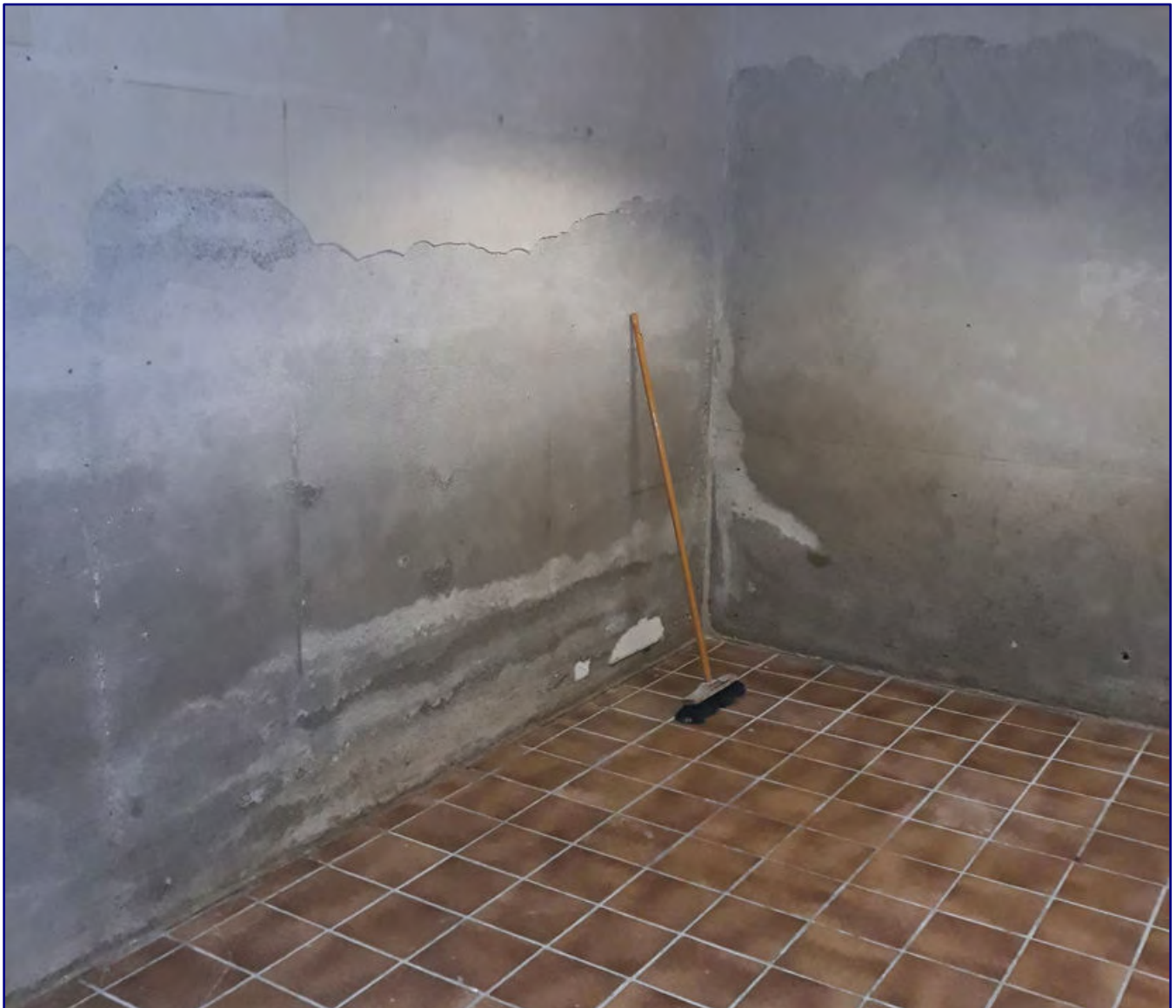
Trafofuchs got off lightly during the flood, but the private rooms and workshop in Erfstadt were damaged. Necessary repairs now hinder ongoing production and require customers to wait longer. Photo: Trafofuchs
