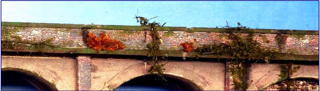
The brick look is also used for the parapet walls. In this way, the structure of the pillars is repeated to a certain degree.
