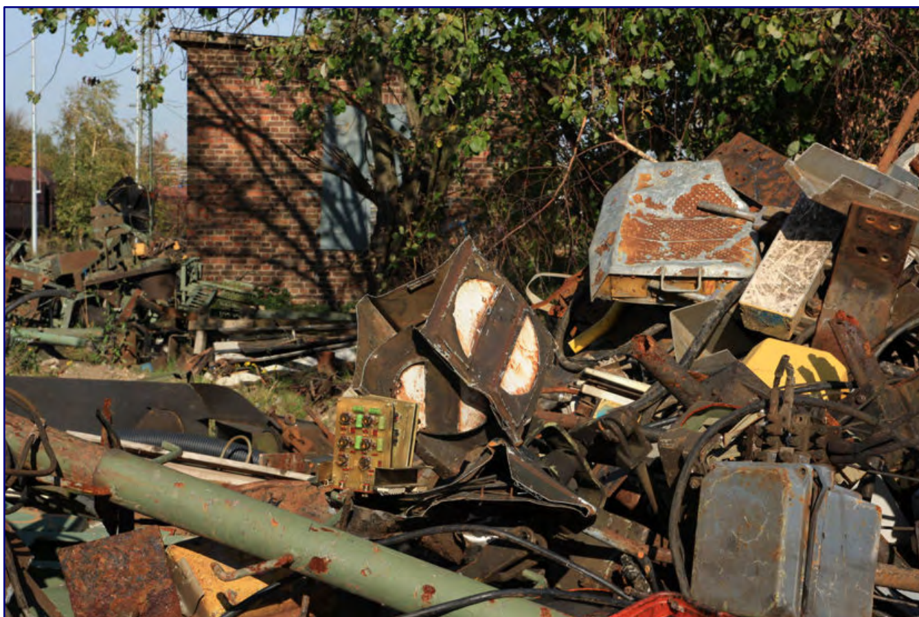
The demolition of the northern workshops, usually called Hall 2, is in full swing in 2013 (photo above). The track dismantling and its typical remnants can also be seen here (photo below).
