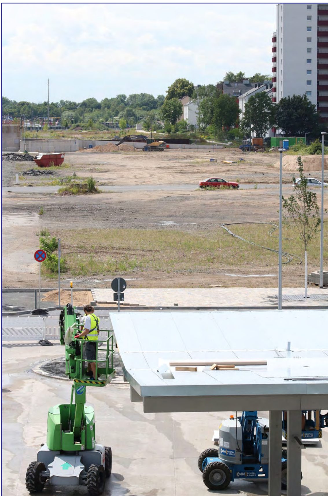
In 2020, nothing could be seen of the old freight tracks any longer; in the foreground, work is underway on the new bus station.
