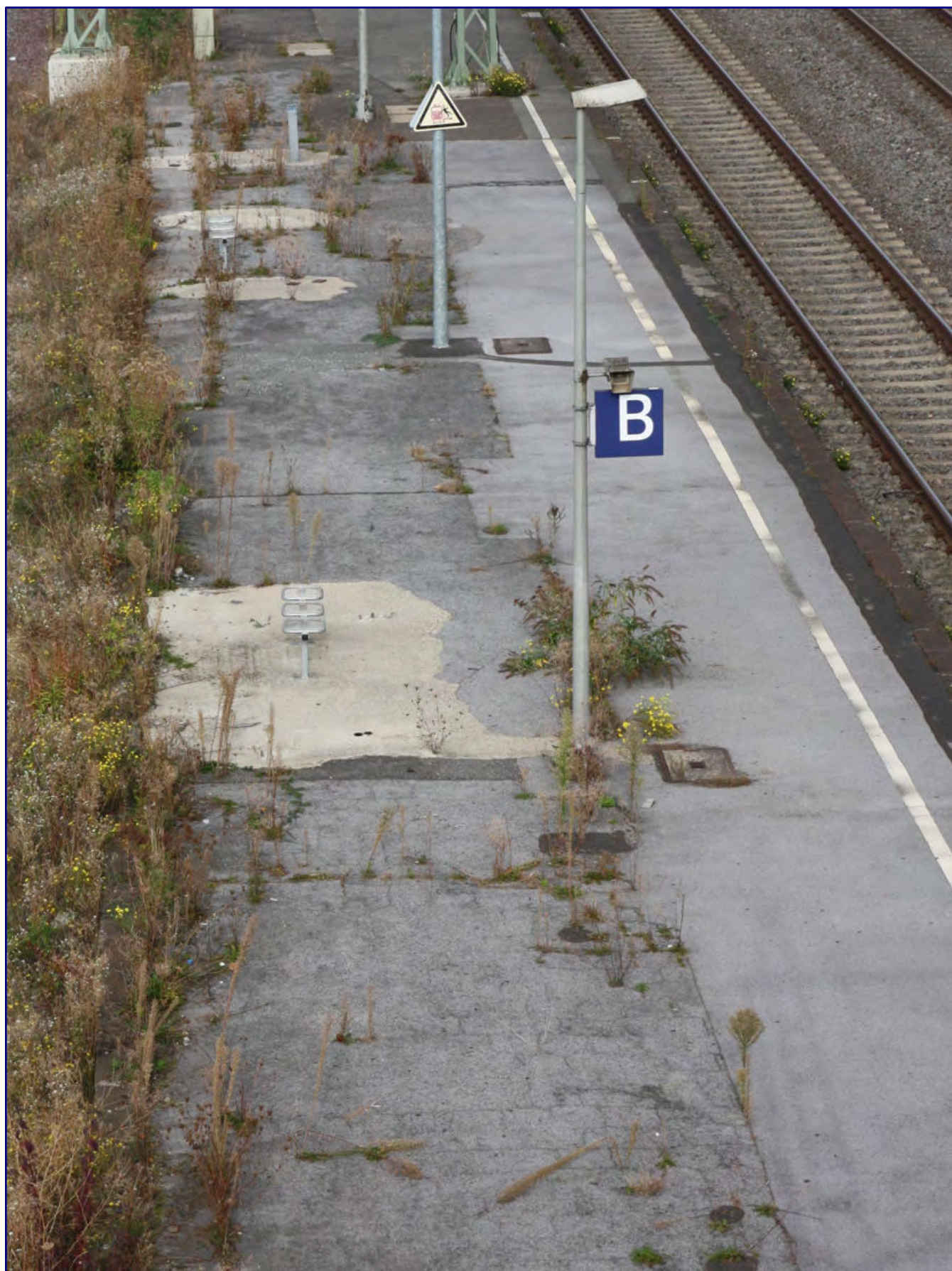
Remnants of the old platform 1 are still present in 2022, unfortunately, not accessible.
