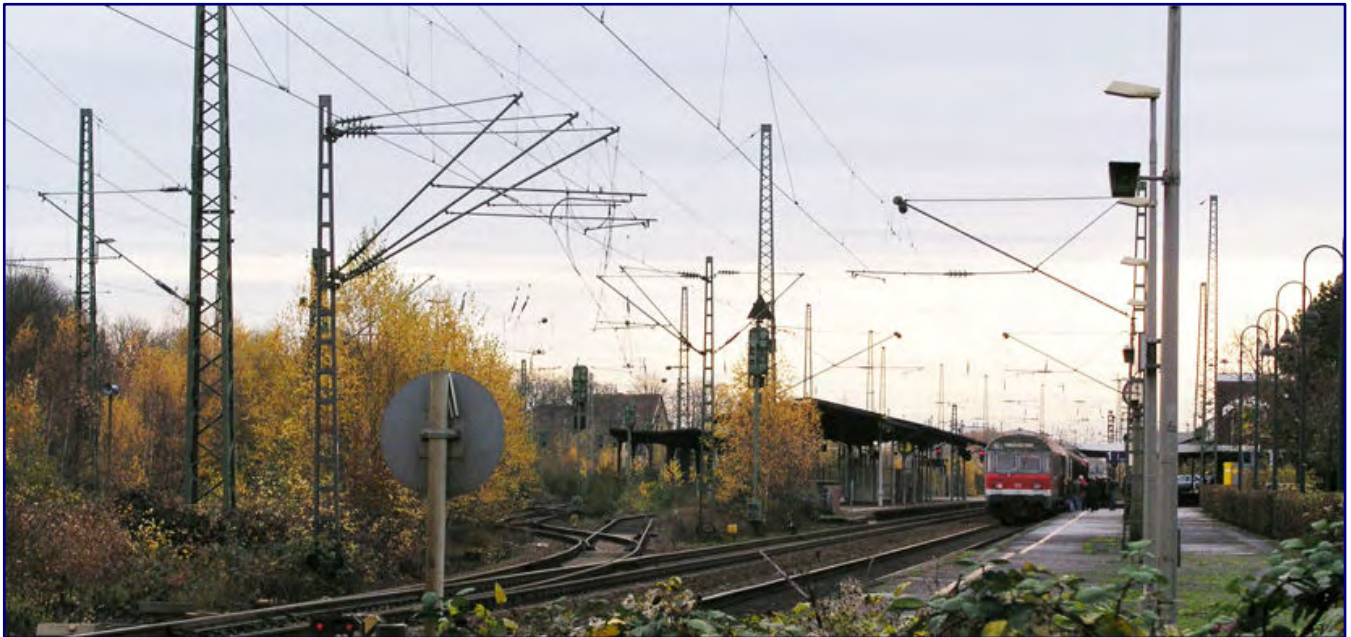
In 2006, the Opladen station area was visibly deteriorating. The Mehdorn era showed the ugly face of the effects of the rigorous austerity mandate at the DB AG during these years.
