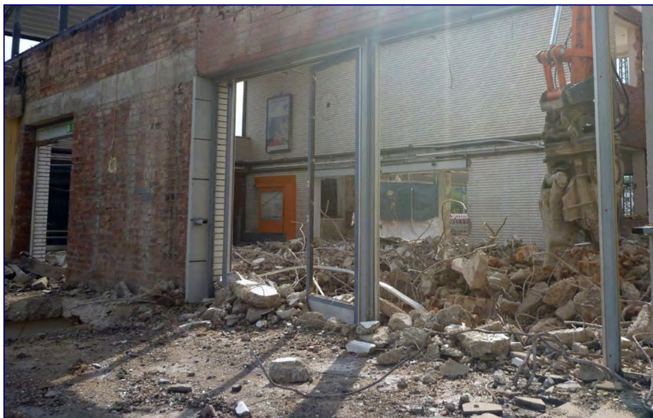
The familiar view for the people of Opladen before going to platform 1 (photo above). This was finally over on 3 September 2015. Opladen no longer had a station building (photo below).
