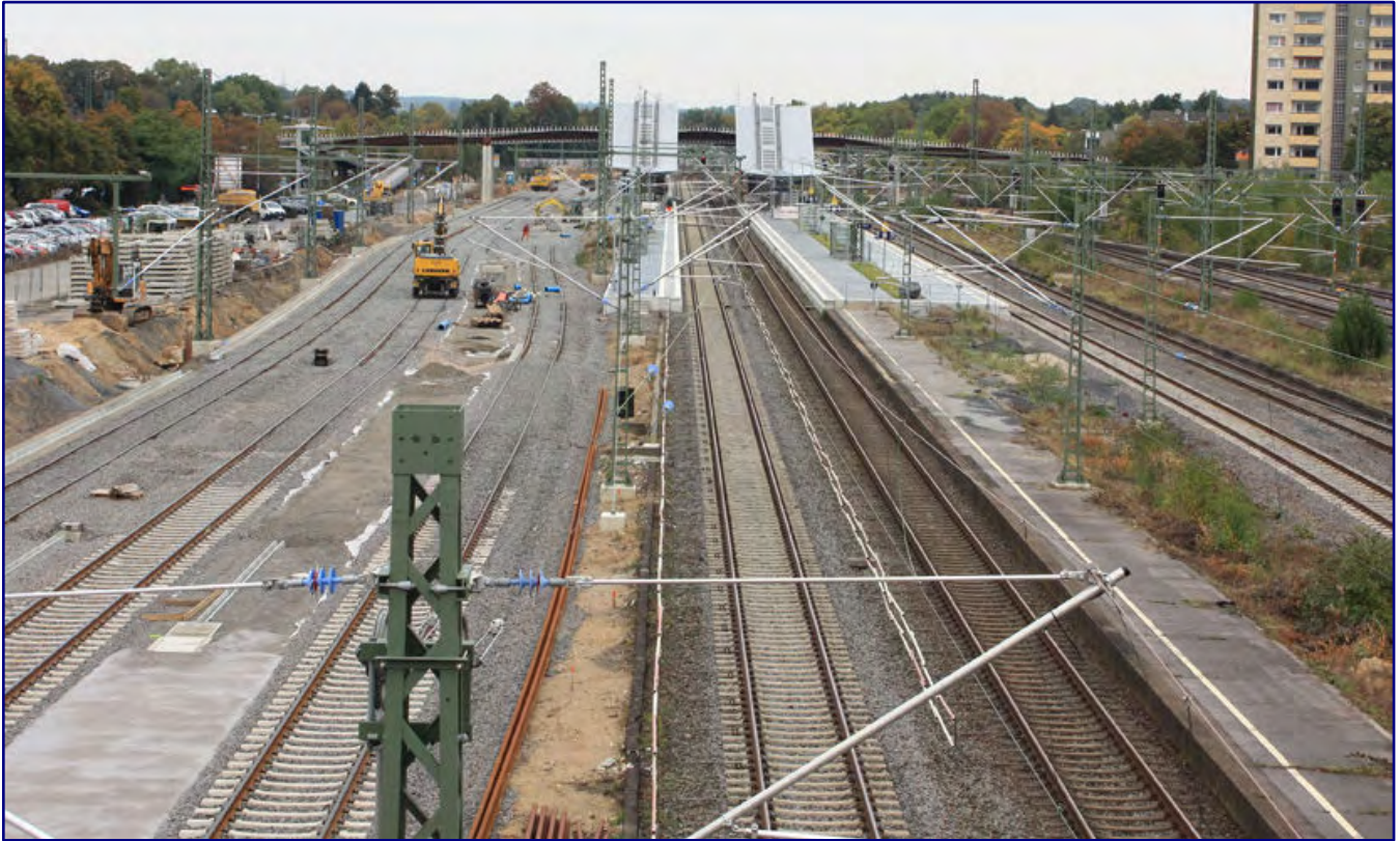
After demolition of the old railroad buildings, work on the new cargo tracks is proceeding at full speed in 2016. The new Opladen station, more of a stopping point, is already in place.
