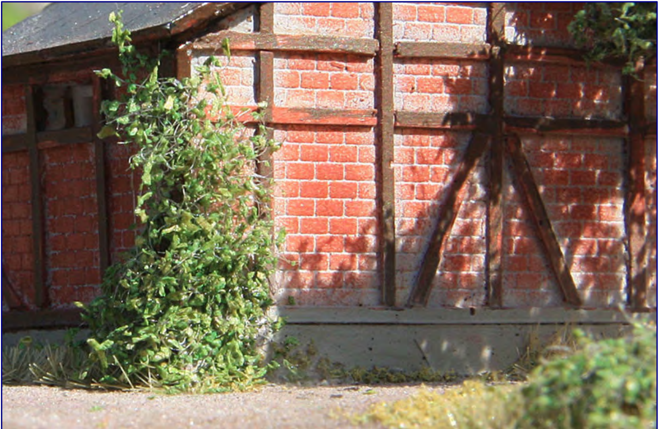
If a house is not maintained, nature will soon take over from all sides.
