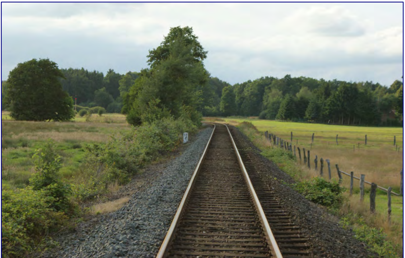
A railway line does not always run through such flat land and manage with such a comparatively low embankment.
