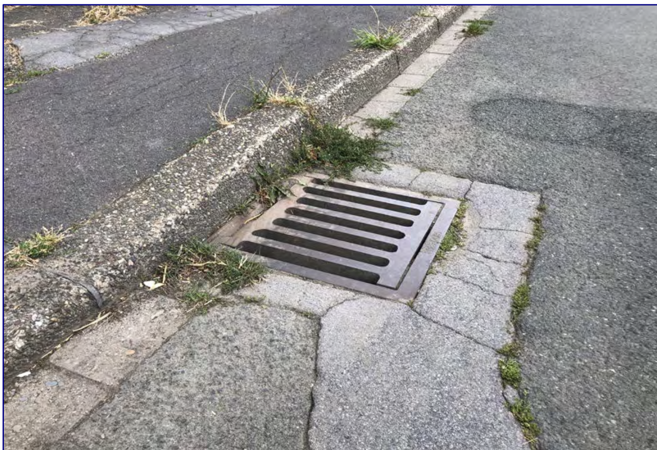
Two examples of cracks and patches in the asphalt are intended to inspire reproduction on the model railway. At the same time, they show how nature is returning. Equally important are the use of manholes (photo above) as well as drainage covers (photo below).
